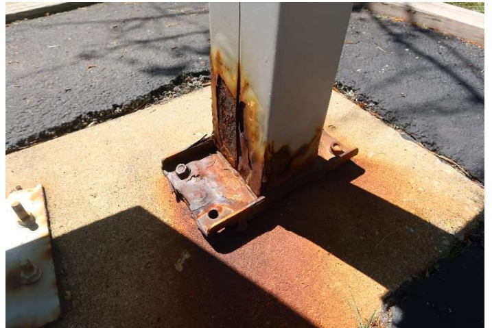
Corrosion at mailbox station base
