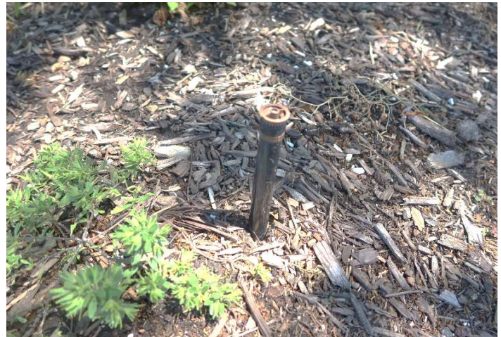
Irrigation head at monument sign
