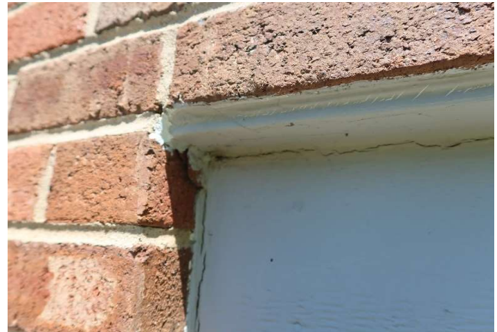
Sealant erroneously located above metal lintel
