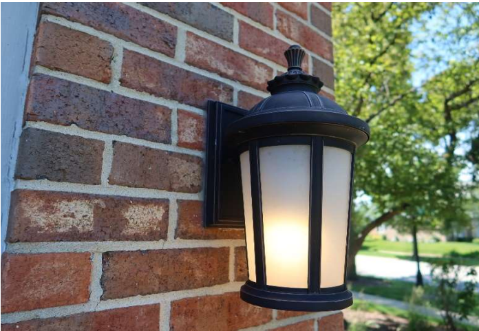
Light fixture overview
