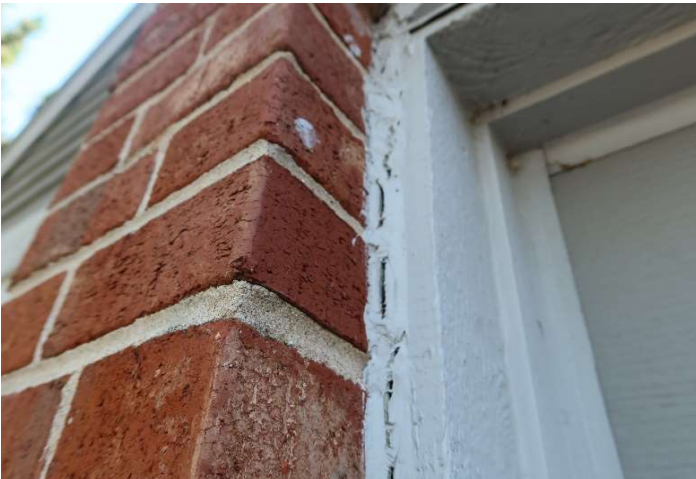
Instance of separated sealant
