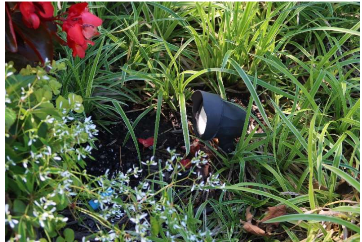
Typical light fixture at monument sign
