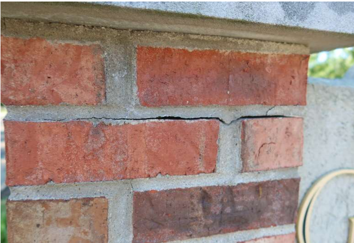
Cracked mortar at monument sign
