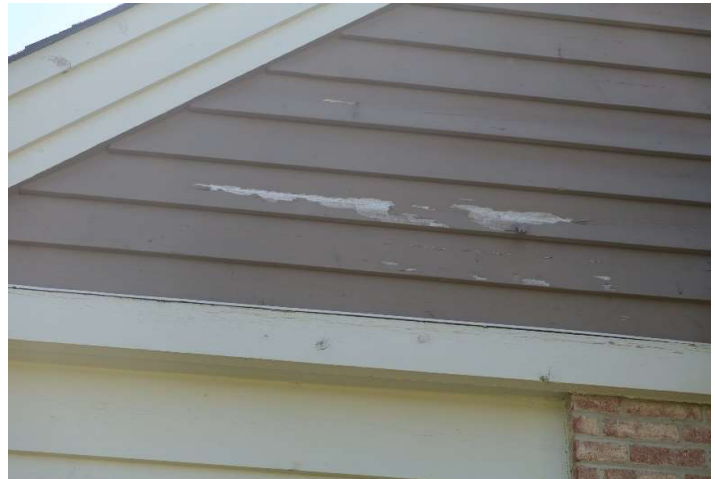
Damaged finishes at wood siding
