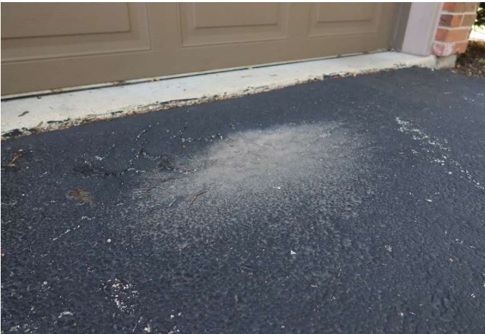
Instance of settlement at asphalt driveway
