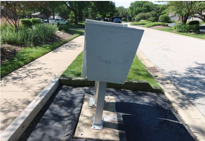
Evidence of leaning mailbox station
