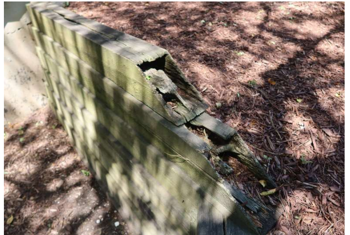
Rotted timbers at retaining wall
