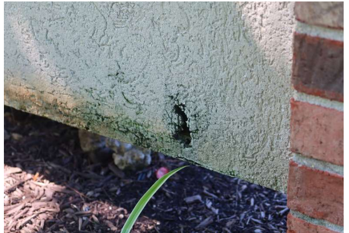
Damage at monument sign
