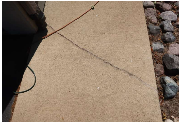
Cracked section of concrete sidewalk
