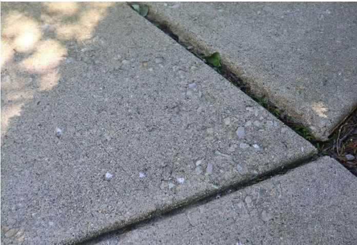
Spalling at concrete sidewalk
