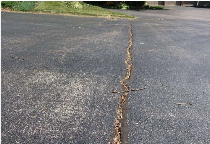
Large crack at asphalt pavement
