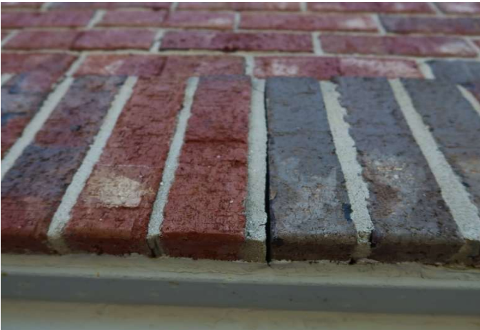
Cracked mortar above garage door
